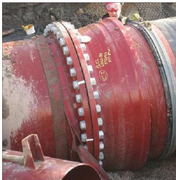
The large pipes needed to transport flows at Fleetwood are subject to huge operating pressures
